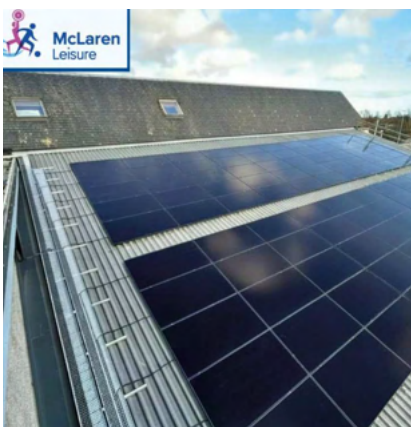
The new solar panels
